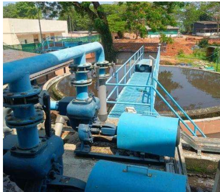
500 KLD STP at Kozhikode medical College
