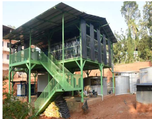
1 MLD STP at Kozhikode medical College
